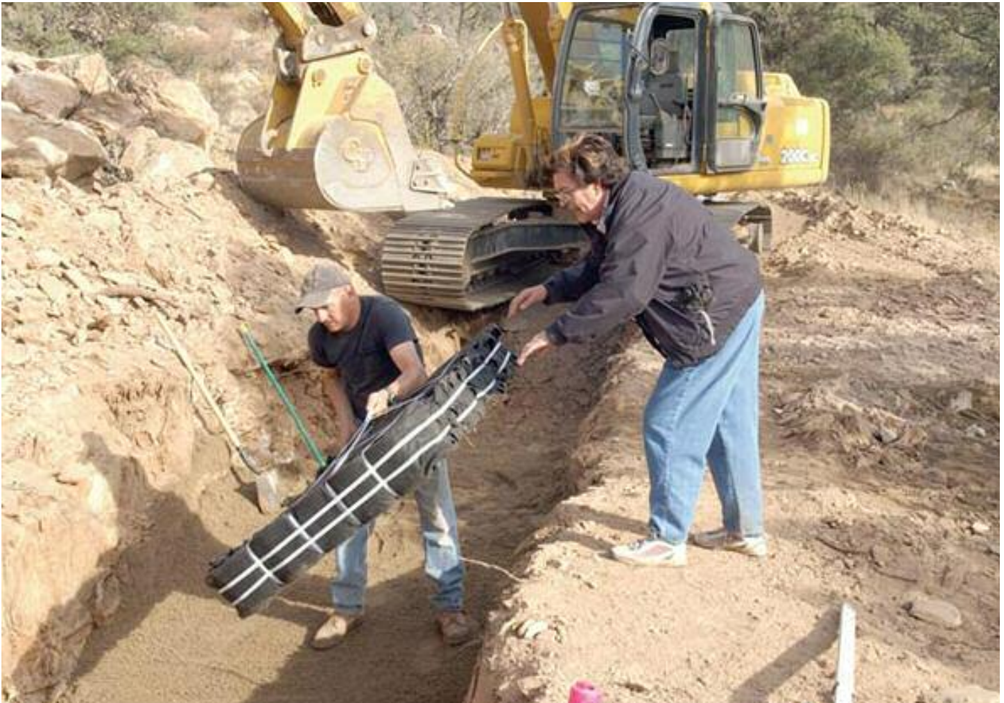
Don Nelson, left takes a filtration section from Lou Brown of Southwest Alternatives as they install an alternative septic system in Crossroads Ranch.
